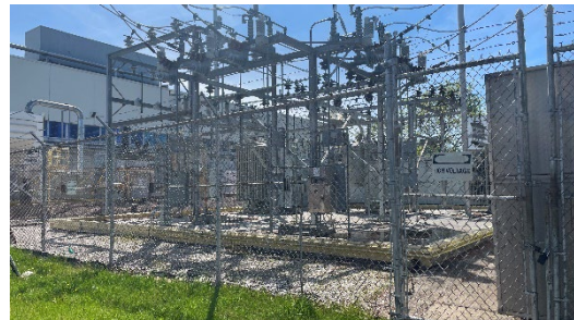
Electrical substation in rear of ATC
