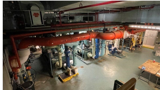
Utility systems in Research Tower basement
