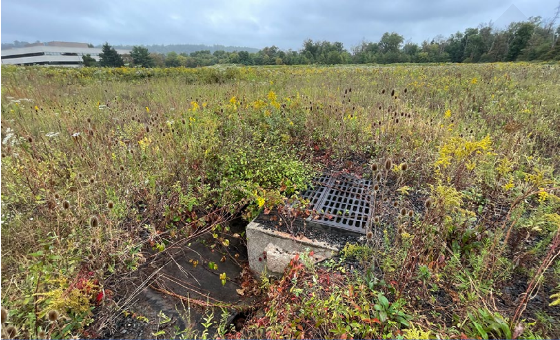
Photo 7. Stormwater Inlet in Gravel Area (Lot 1.04)
