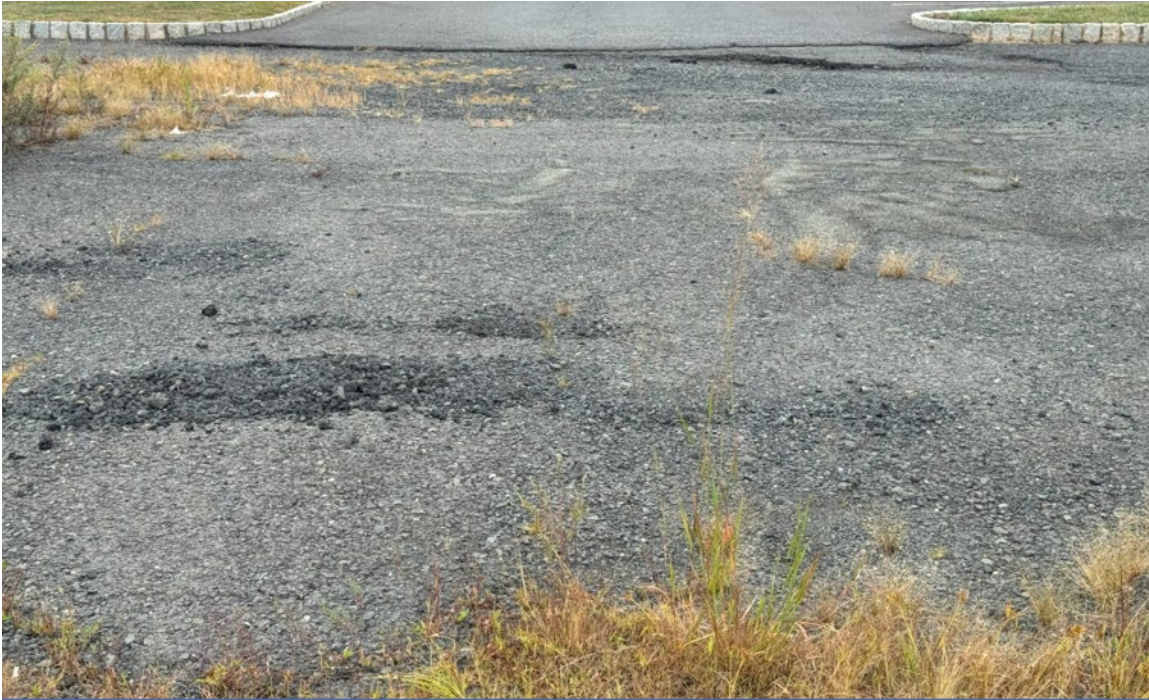
Photo 25. Degrading Asphalt Pavement (Lot 1.04)
