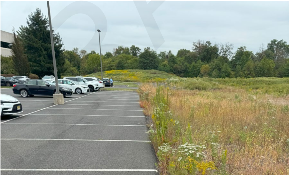
Photo 28. Pavement Edge with No Curb (Lot 1.04)
