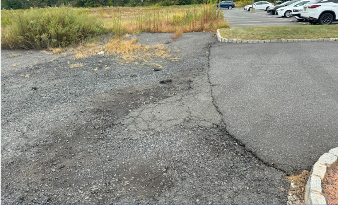
Photo 19. Degradation of Asphalt Pavement (Lot 1.04)
