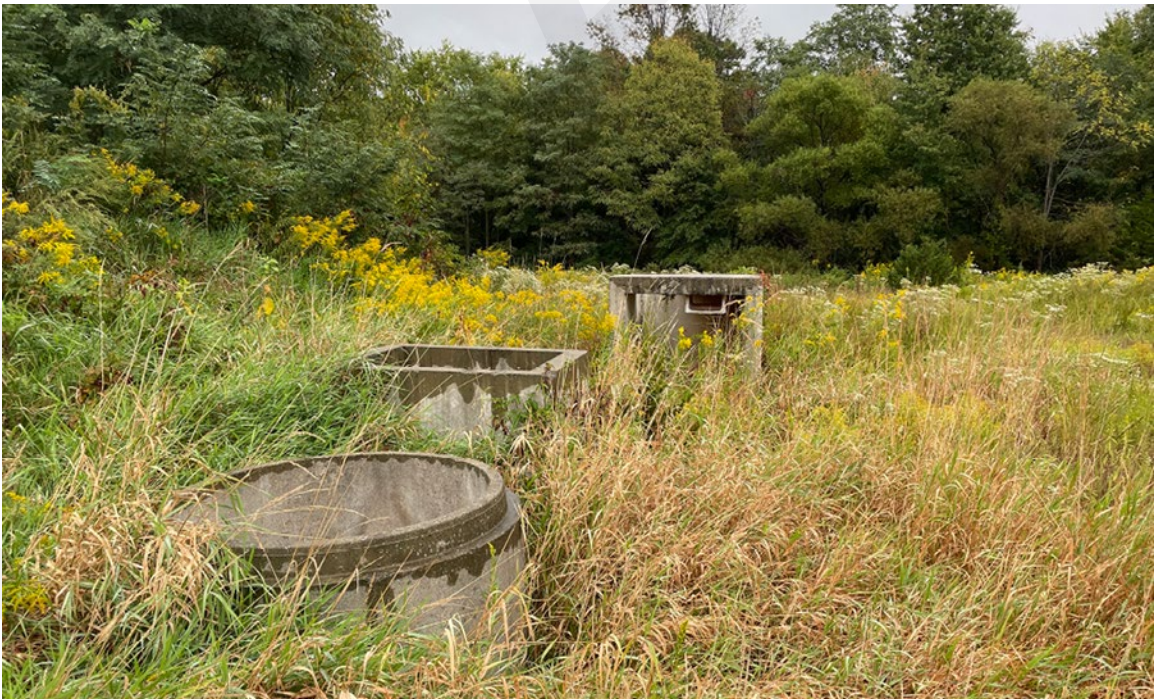
Photo 10. Unused Stormwater Management Components (Lot 1.02)
