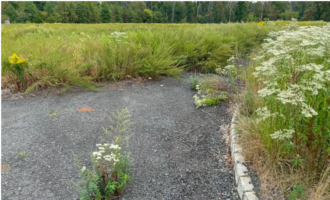
Photo 26. Pavement Edge with No Curb (Lot 1.02)
