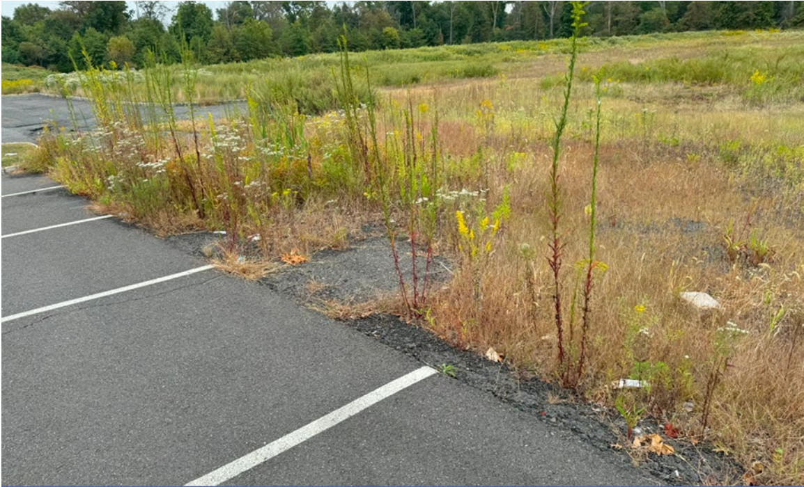
Photo 27. Pavement Edge with No Curb (Lot 1.04)
