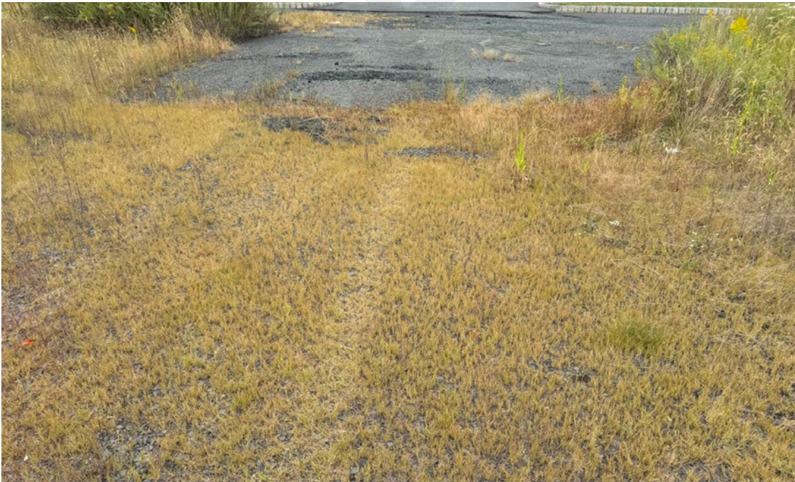
Photo 17. Exposed Gravel Base with Vegetation
